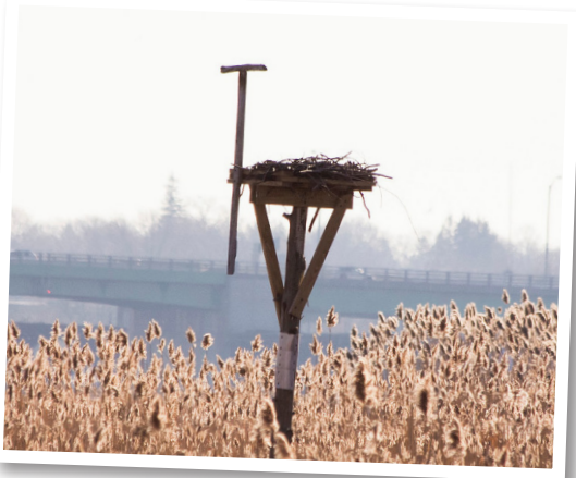
MSEC STUDENTS AT THE MERRIMACK VOCATIONAL HIGH SCHOOL BUILT THIS 16 FOOT "OSPREY POLE" AND INSTALLED IT ON AN ISLAND IN THE MERRIMACK RIVER.
